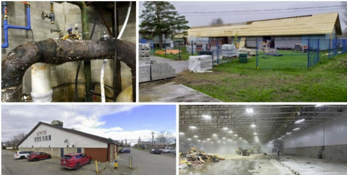
Facilities in Kemptville and Arnprior. Across the country, aging pools, rinks, and community centres—most built during Canada's centennial era—are falling apart, writes Martin Sampson. Photograph courtesy of Canadian Parks and Recreation Association
